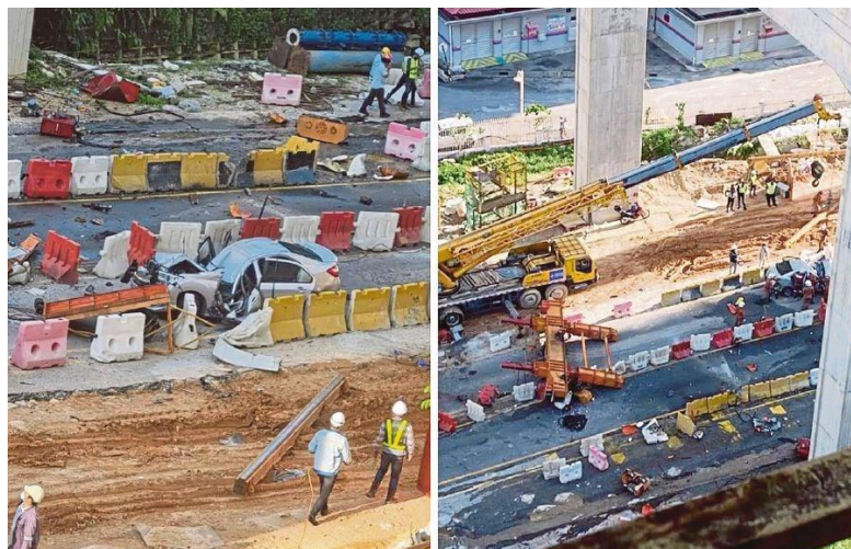
Figure 1: Accident Occurred on the Sungai Besi-Ulu Kelang Elevated Expressway (SUKE)
